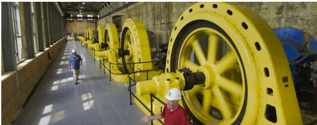
Mechanicville Hydroelectric Plant is the longest-running hydro plant in the U.S. and one of the oldest in the world. Source: Paul Buckowski/Albany Times Union
